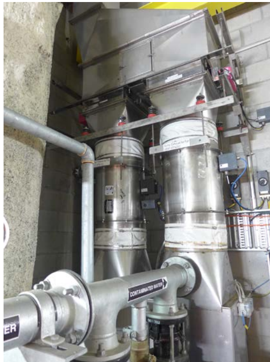
Figure 2-13: Tunnel sump ventilation system in the Victoria Park Tunnel.
