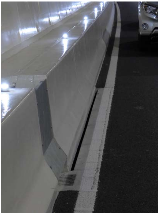
Figure 2-9: Example of a slot drain in the Waterview Tunnel.
