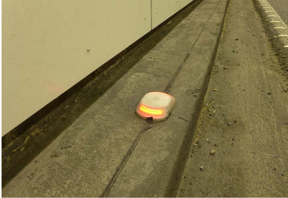
Figure 2-64: Mount Victoria Tunnel roadway marking lighting and slot for power.
