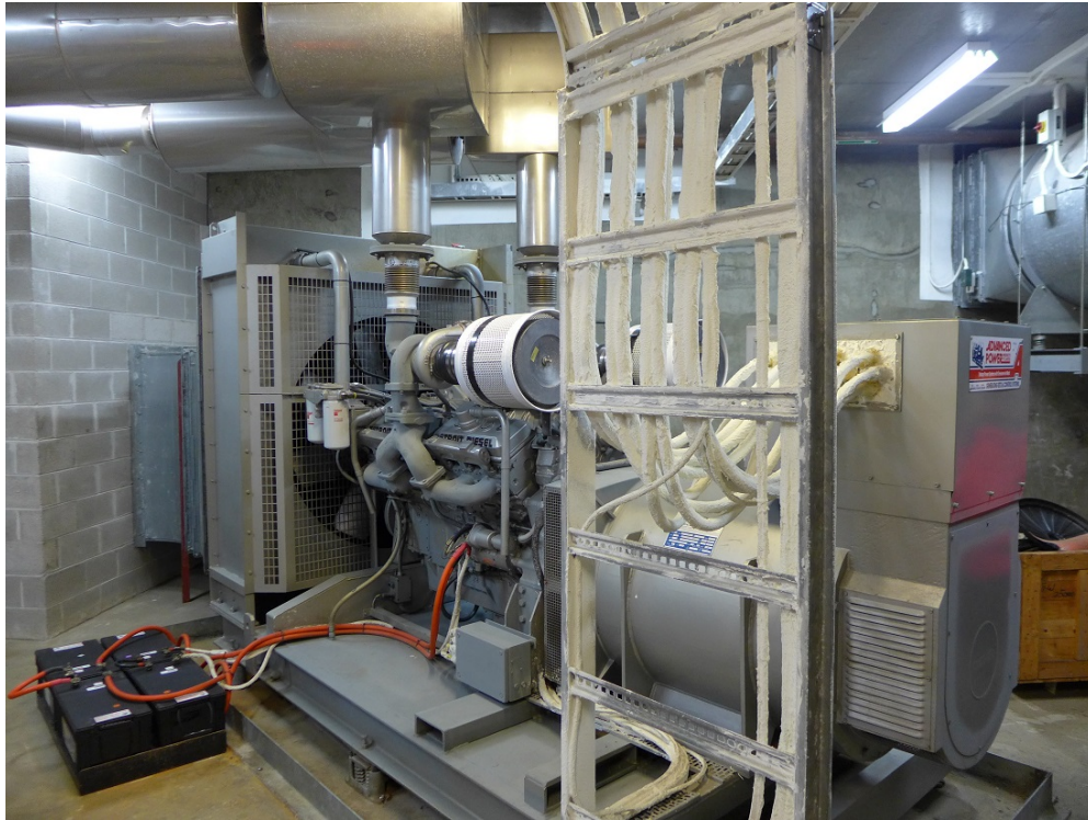
Figure 2-68: Cables coated in fire proofing material, located next to a generator, Sydney Harbor Tunnel.
