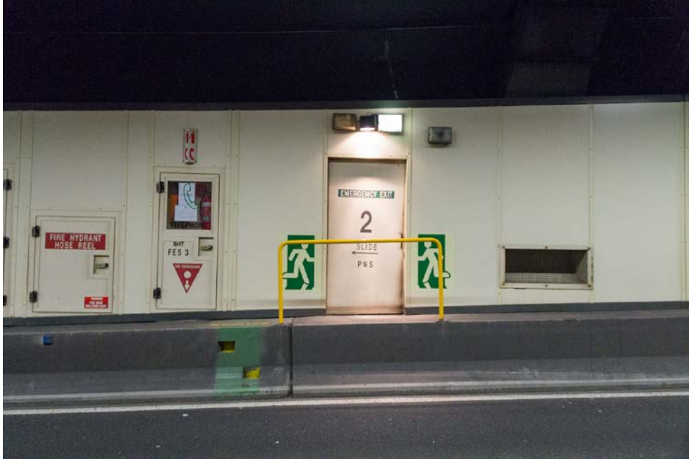
Figure 2-61: Sydney Harbor Tunnel emergency exit signage.
