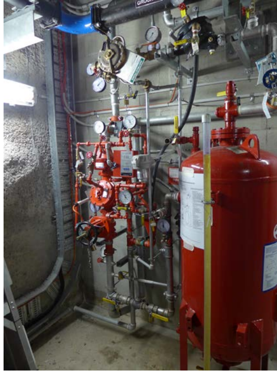
Figure 2-12: Foam suppression system for a tunnel sump in the Victoria Park Tunnel
