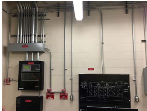
Figure 2-67: Typical U.S. tunnel cable arrangement with conduit (photo opportunity courtesy of Caltrans).
