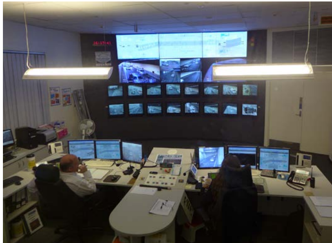
Figure 2-37: Sydney Harbor Tunnel control room.
