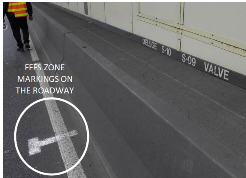
Figure 2-17: Road markings of FFFS zone boundaries in the Sydney Harbor Tunnel.
