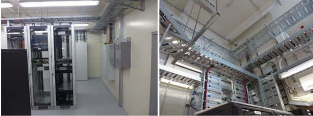
Figure 2-66: Cable arrangements in the Mount Victoria and Terrace Tunnel electrical spaces.
