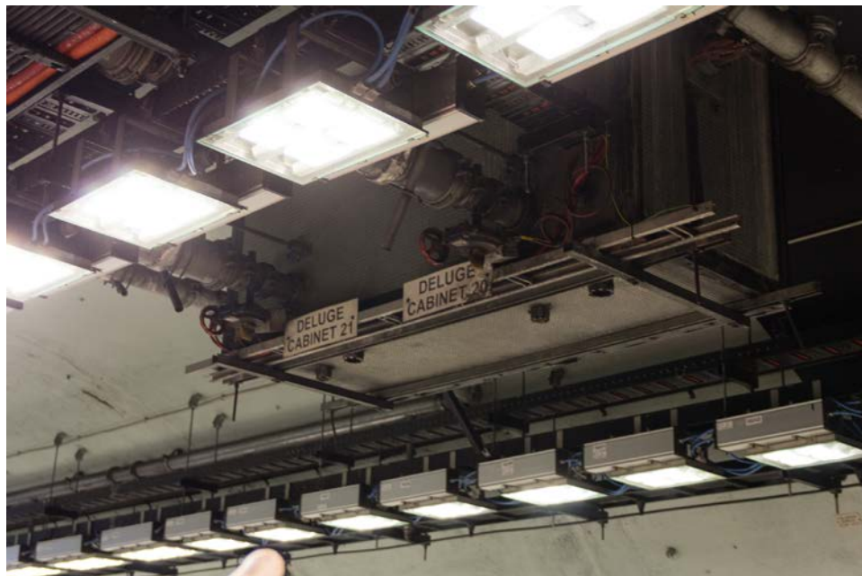
Figure 2-28: Mount Victoria Tunnel close-up of FFFS (deluge) valve in the tunnel apex.
