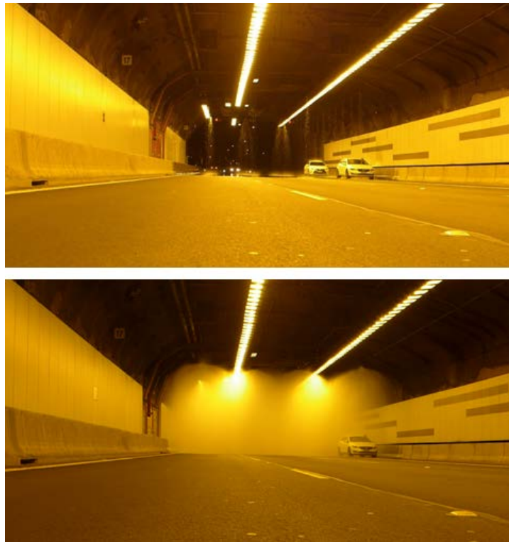
Figure 2-36: M2 tunnel with no FFFS activated (top) and FFFS activated (bottom)
