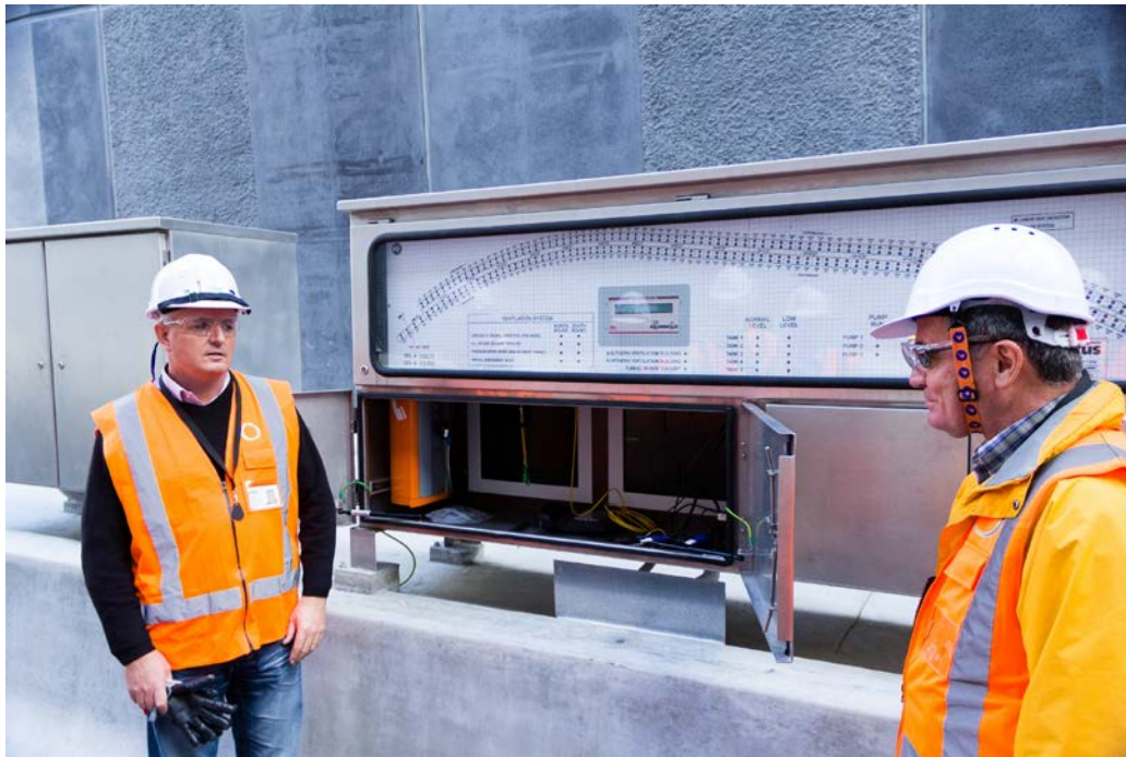
Figure 2-14: Waterview Tunnel fire command post showing screens for incident playback to the response crew.
