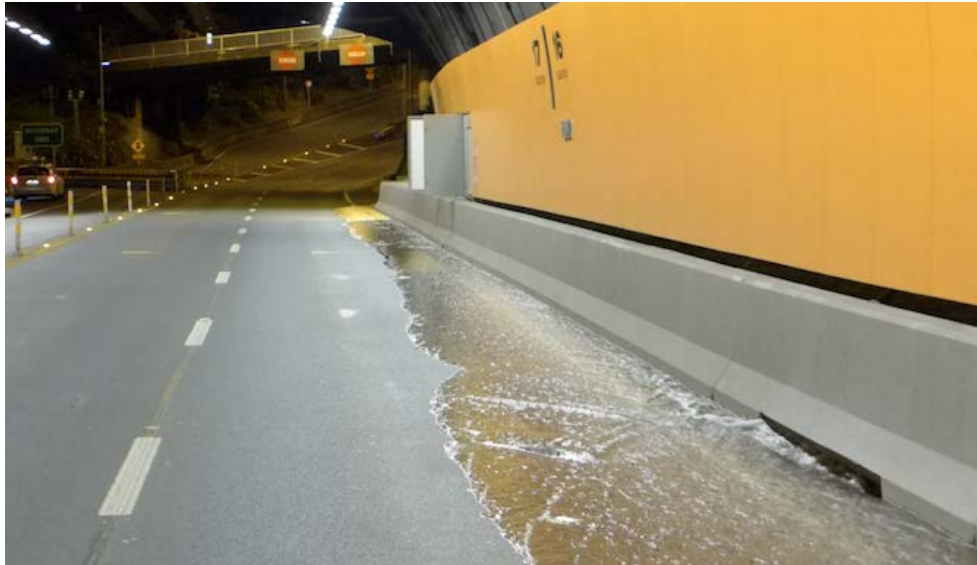
Figure 2-10: Water overflowing a drain in the Terrace Tunnel during an FFFS test.
