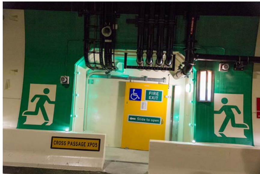
Figure 2-59: Waterview Tunnel exit signage at cross passage egress door.
