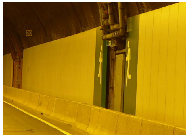
Figure 2-3: M2 Tunnel, cross passage with FFFS branch pipework above door.
