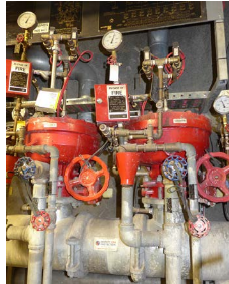
Figure 2-2: M2 Tunnel, FFFS zone (deluge) valves.
