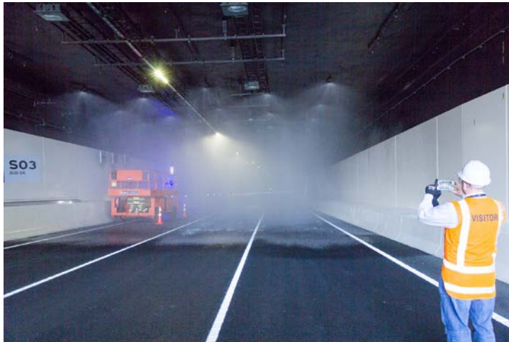
Figure 2-29: Waterview Tunnel demonstration of the FFFS operation.
