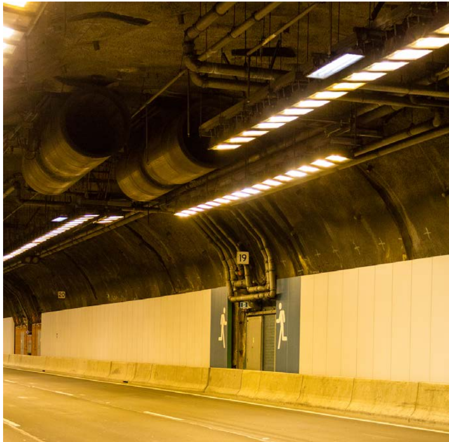
Figure 2-62: M2 Tunnel emergency exit signage.
