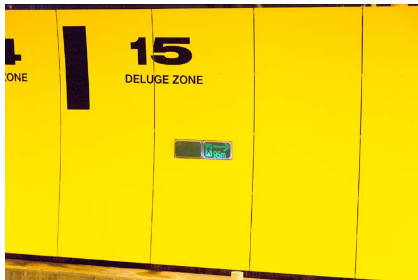
Figure 2-60: Terrace Tunnel with lit directional exit signage on walls.
