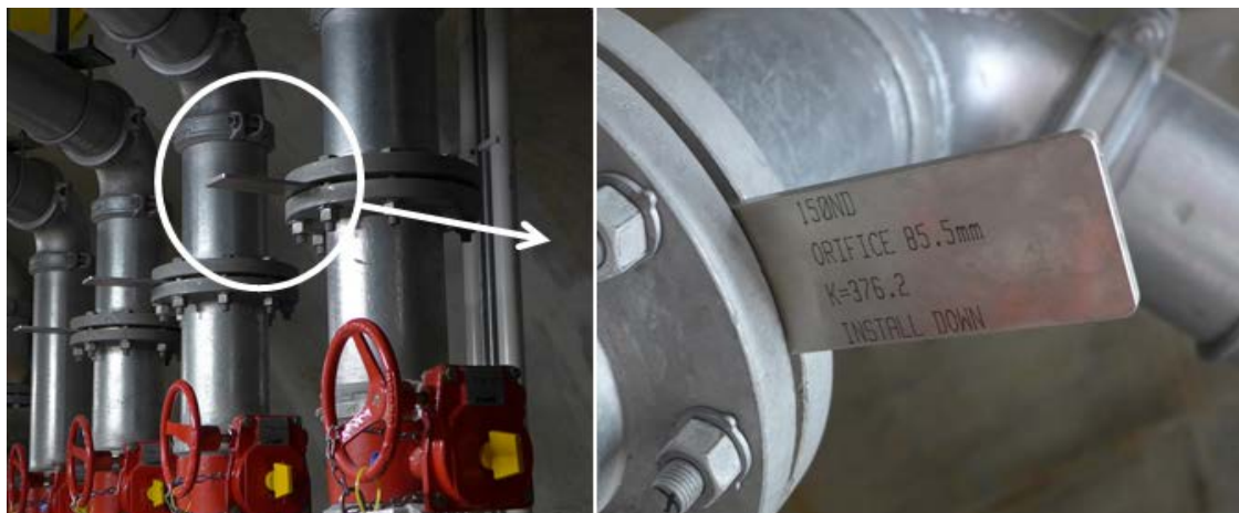
Figure 2-30: Waterview Tunnel FFFS valve with orifice plate.
