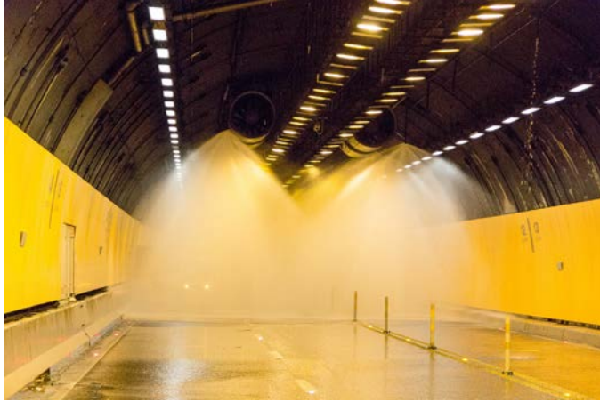
Figure 2-4: FFFS activation in the Terrace Tunnel at water application rate of 0.16 gpm/ft 2 (6.5 mm/min).
