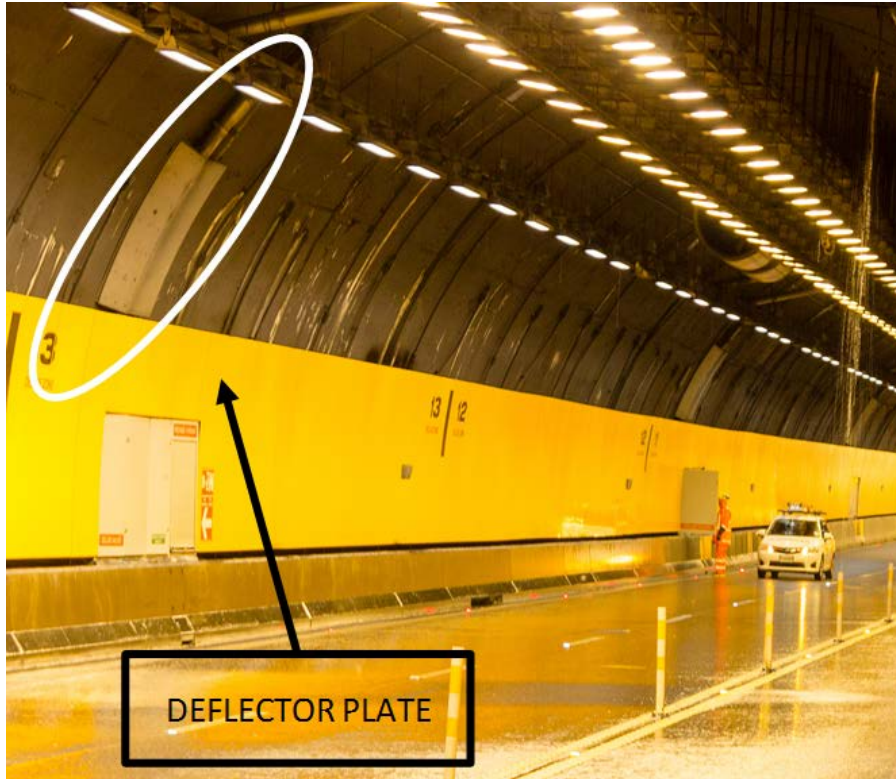
Figure 2-22: Deflector plate installed on the Terrace Tunnel branch main to overcome minor traffic envelope overlap.
