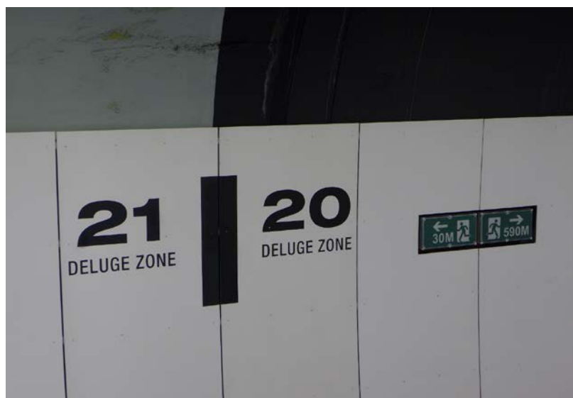
Figure 2-18: FFFS zone markings on the wall in the Mount Victoria Tunnel.
