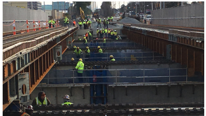
FIGURE 4. BRIDGE SLIDE, NORFOLK SOUTHERN RAILROAD OVER I-240, MEMPHIS, TENNESSEE. THE BRIDGE ELEMENTS WERE BUILT ADJACENT TO THE EXISTING BRIDGE. SOURCE: FHWA
