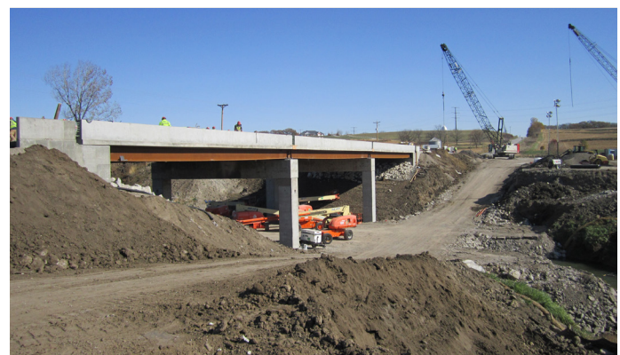
FIGURE 2. KEG CREEK BRIDGE REPLACEMENT, COUNCIL BLUFFS, IOWA. PREFABRICATED BRIDGE ELEMENTS WERE TRANSPORTED AND ERECTED IN PLACE USING CRANES IN ABC. SOURCE: IOWA DEPARTMENT OF TRANSPORTATION
