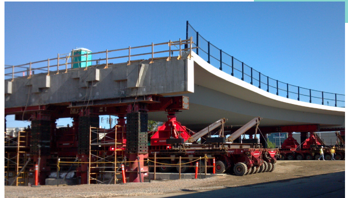
FIGURE 3. PREFABRICATED BRIDGE, PECOS STREET. BRIDGE OVER I-70 AND PECOS, DENVER, COLORADO. BRIDGE ELEMENTS WERE BUILT NEAR THE SITE, LIFTED WITH HYDRAULIC JACKS, AND MOVED INTO PLACE USING SPMT. THE BRIDGE WEIGHED 2,400 TONS AND TOOK 50 HOURS TO MOVE A DISTANCE OF 800 FEET. SOURCE: FHWA
