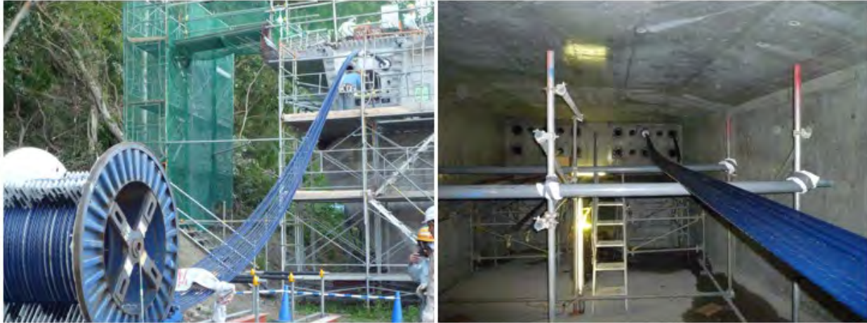
Figure 20: Epoxy-coated strand being unwound and pulled through the ducts during construction. (Source: Sumiden Wire Products)
