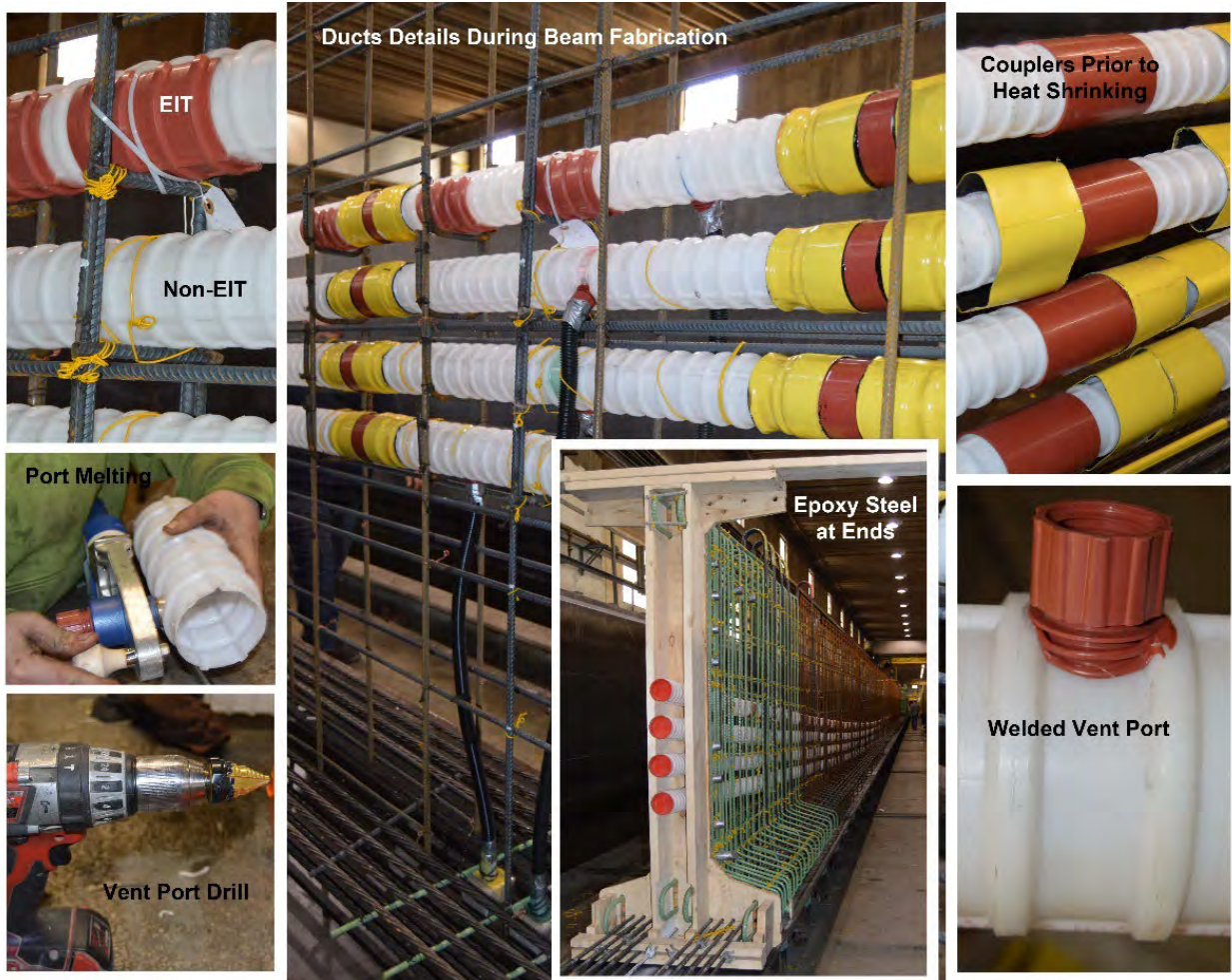
Figure 4: The various ducts and ports necessary for the implementation of the electrically isolated tendons. (Source: Dr. Clay Naito)
