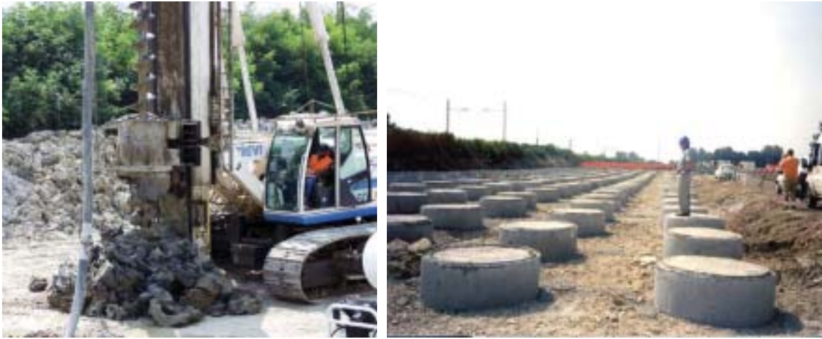
Figure 14. CFA pile-supported embankment project for the high-speed rail project: (a) CFA pile installation and (b) installed CFA piles.
