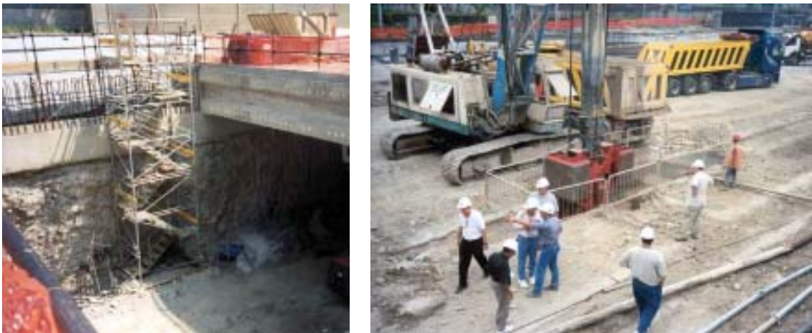
Figure 15. Turin subway project site visit showing: (a) station excavation and (b) continuous diaphragm wall construction.
